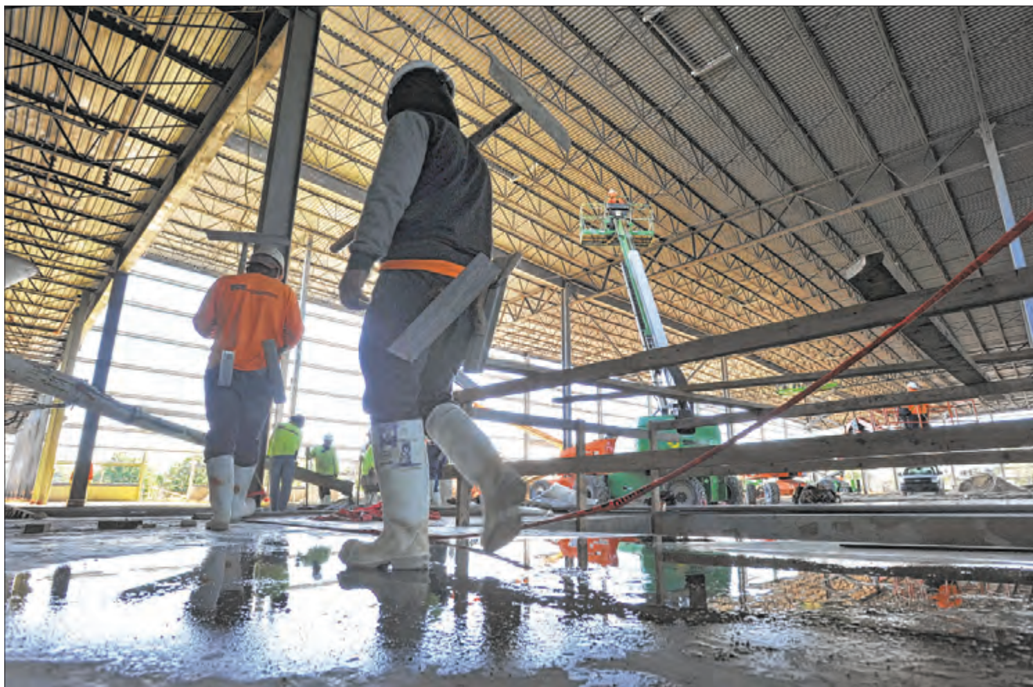
Workers continue construction of the new Ikea store Thursday in Jacksonville. (Will Dickey/Florida Times-Union)
