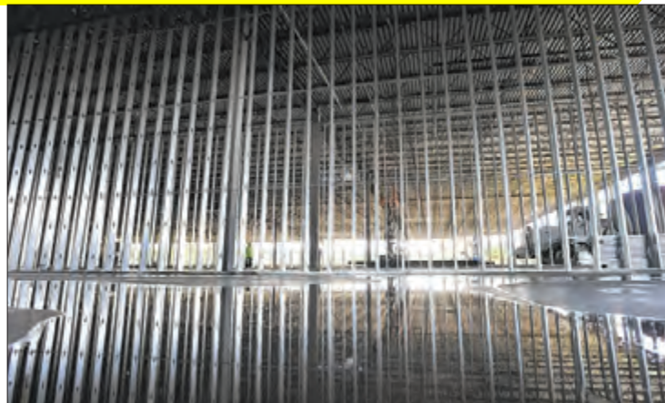
Structural studs reflect in water from the previous night's rainfall during construction at the new Ikea home furnishings store at Gate Parkway and I-295 Thursday. (Will Dickey/Florida Times-Union)
